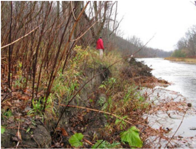
Photo 4.1-7 Bank failure on West Seneca Developmental Center site along Cazenovia Creek with Japanese knotweed riparian understory
